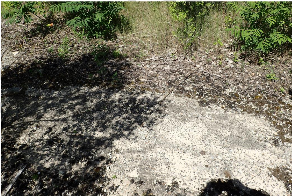
Photo 10: Concrete pavement adjacent to shoreline escarpment looking west.
