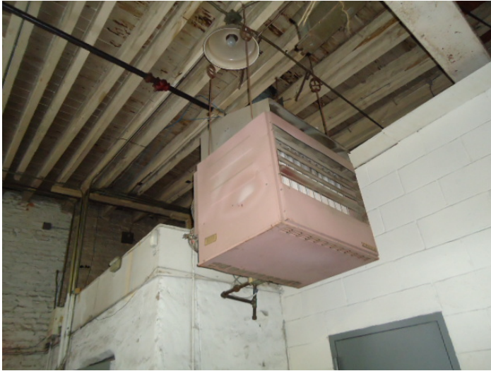
13. Gas-fired ceiling-mounted heater
