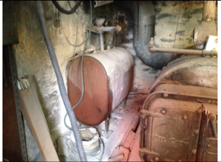
PHOTO 8: Looking at the oil tank associated with the oil fired hot air blower heating system.
