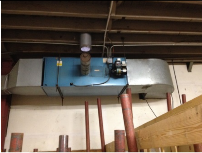
PHOTO 7: Looking at the oil-fired hot air blower heating system.
