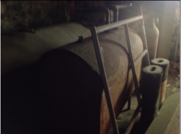
PHOTO 10: Looking at a second 275-gallon AST and behind that is another AST encased within concrete.
