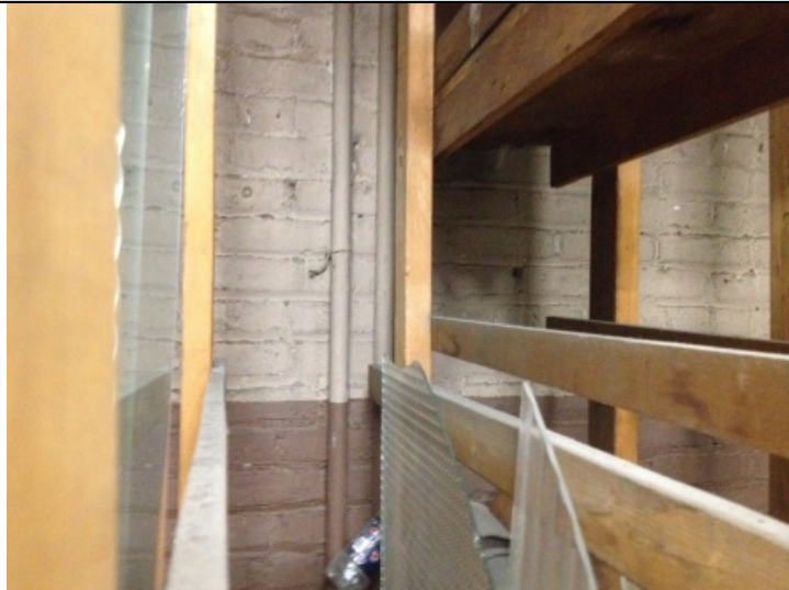
PHOTO 11: Looking at two gas tank vent lines that run up along the front wall of the building.
