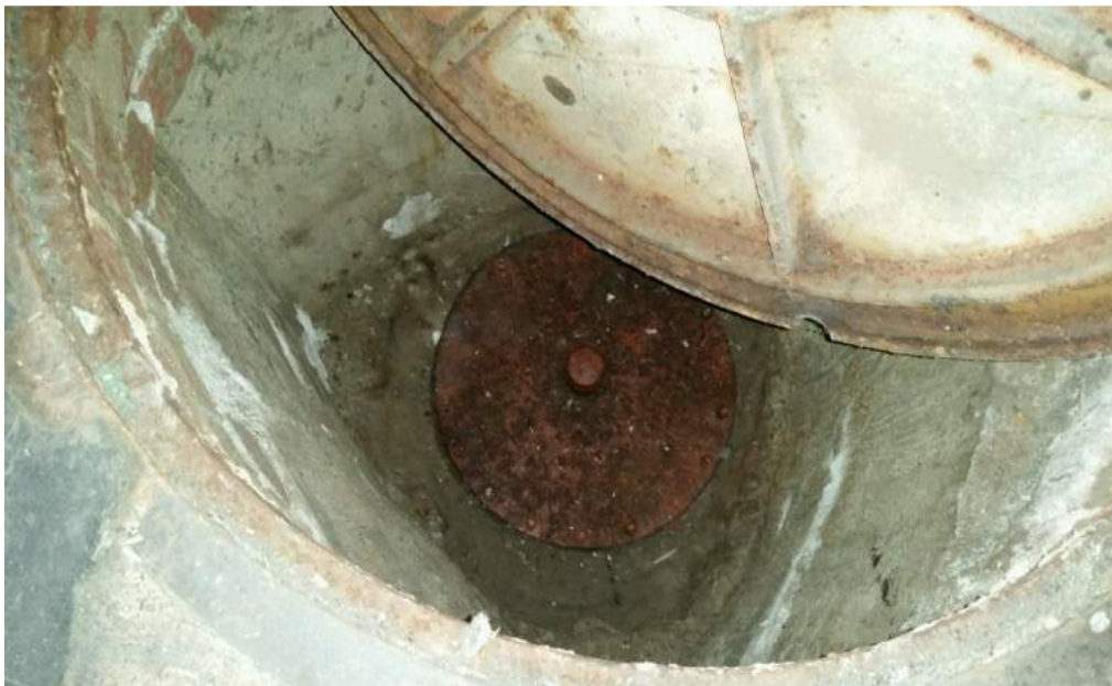
Photo 2: View of the potential tank beneath the non-descript manhole in the southeastern room
