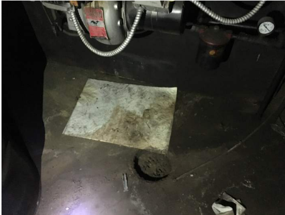
Photo 9: View of a stained absorbent pad and drain beneath the fuel oil connection pipe to the boiler
