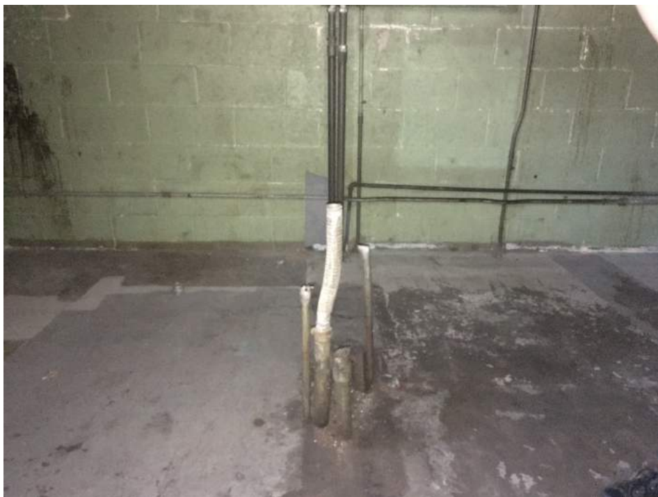
Photo 4: View of former electrical and mechanical connections in the northeastern room on the first floor, facing west
