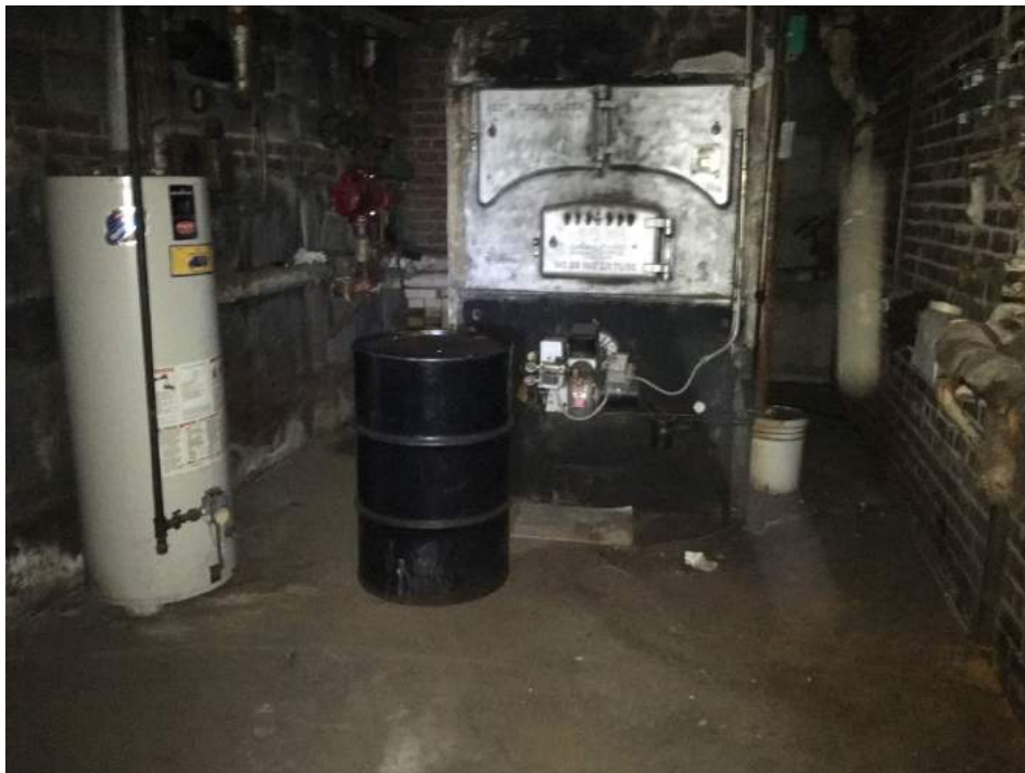
Photo 8: View of the boiler room and 55-gallon drum containing an oily liquid, facing east
