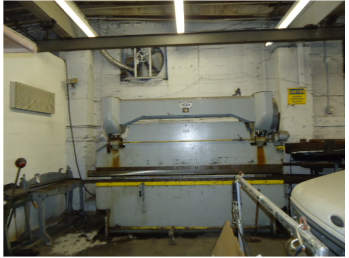
10. Machinery inside building
